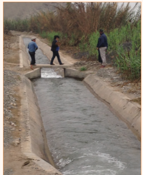
Flume Installed in an Irrigation Channel to Monitor Volume
