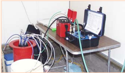
Completed 7 zone installation showing groundwater sampling using a Model 466 Pump Controller and level measurements using a Readout Box.
