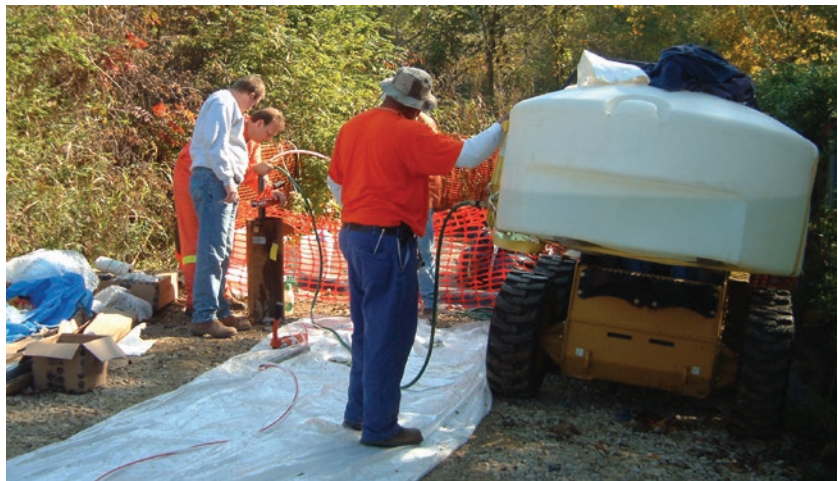
Figure 8-1 Adding Water to the System
