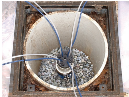
Figure 9-1 Tubing Organized Around the Wellhead
