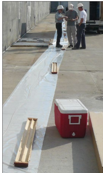
Figure 4-1 Plastic & SS Support Cable Laid Out (Wood core boxes are used here to weigh down plastic)
