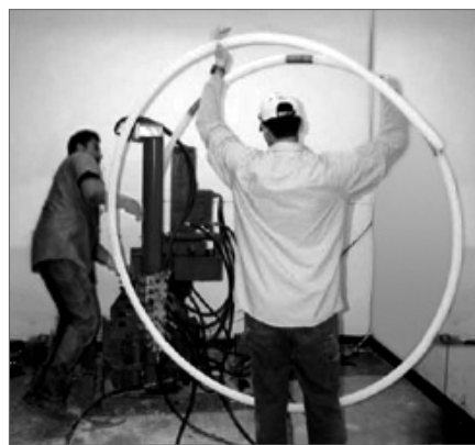
7-Channel CMT installation for monitoring groundwater and soil gas beneath a building.
